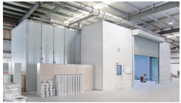
Typical Coating Facilities
