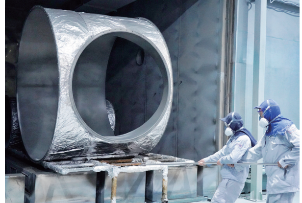
Large Coating Oven
